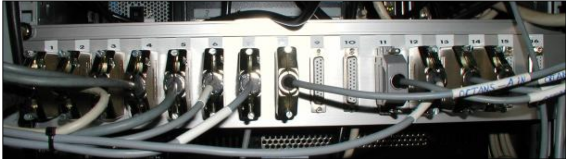
Figure 8: Data Distribution Board
